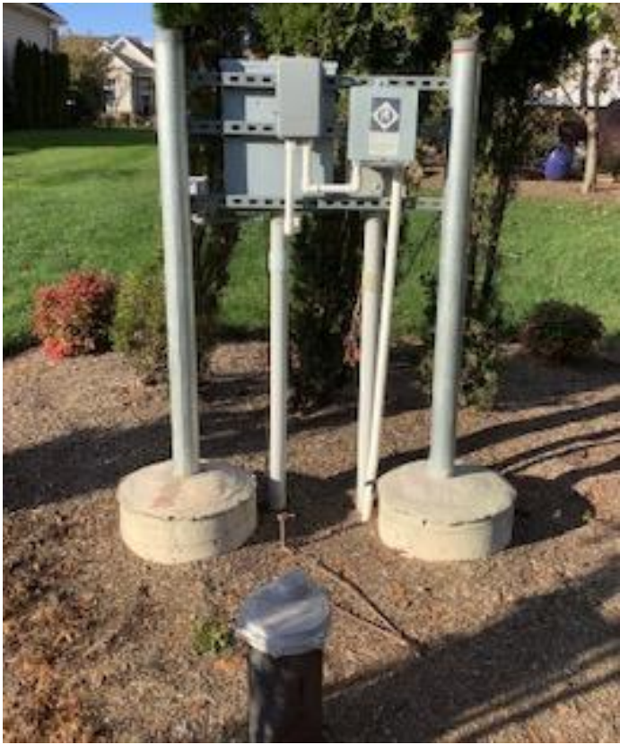
Well site at northwest corner of Pond 4 has electric power panel and well pump controls.
