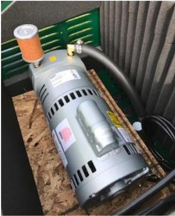
Compressor for bubble aerator system is a Gast rotary vane, model 1023-101Q-G608NEX, rated at 10 cfm, 10 psi.
