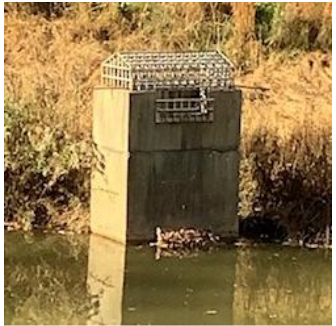
Outlet structure discharges to adjacent wetlands through reinforced concrete pipe.
