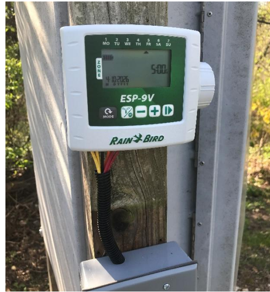
Programmable digital controller located at well site controls daily amount of make-up water to the pond (as well as irrigation water for Sloan clubhouse).
