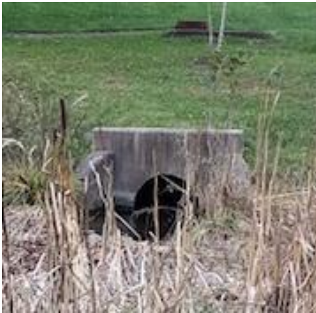
Inlet structure is fed from the Phase 3 storm water systems.
